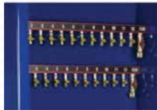
12 1/4" water circuits & one 1/2" circuit for water manifold supply
